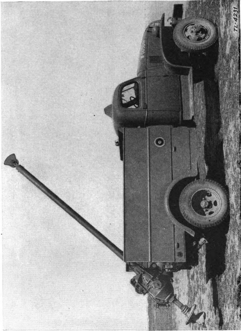
FIGURE 2.—Truck W-44-B with earth borer equipment HD, arranged to bore hole at an angle—side view.
